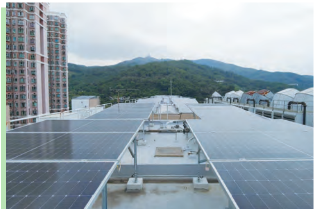
Solar Panels in CDW Building
