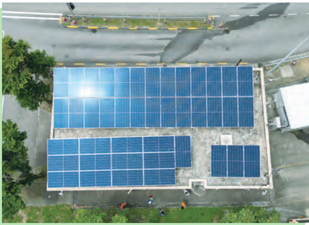
Solar Panels in Discovery Bay Tunnel Building No. 1
