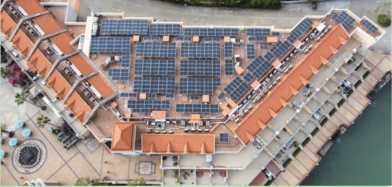
Solar Panels in DB North Plaza
